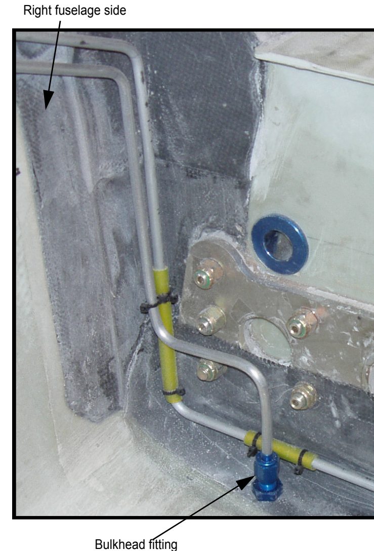
Figure 12.3.H.1 Bulkhead fitting for brake lines from inside the fuselage.
